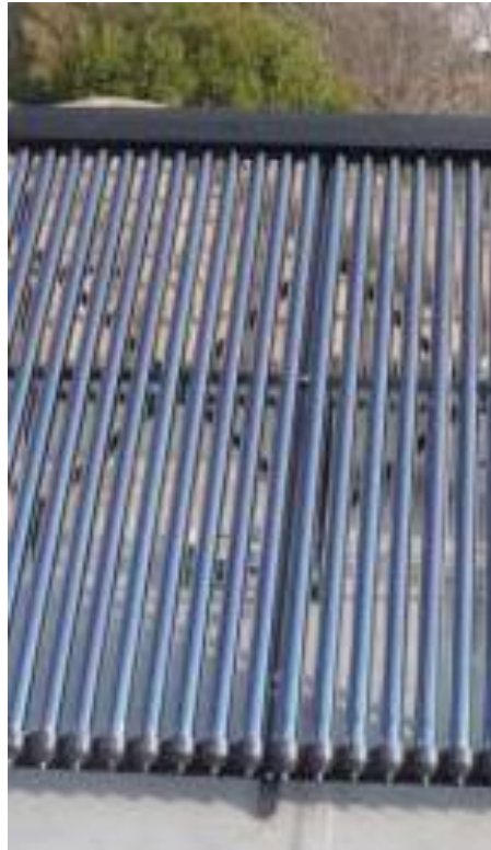
Solar thermal for heat generation
